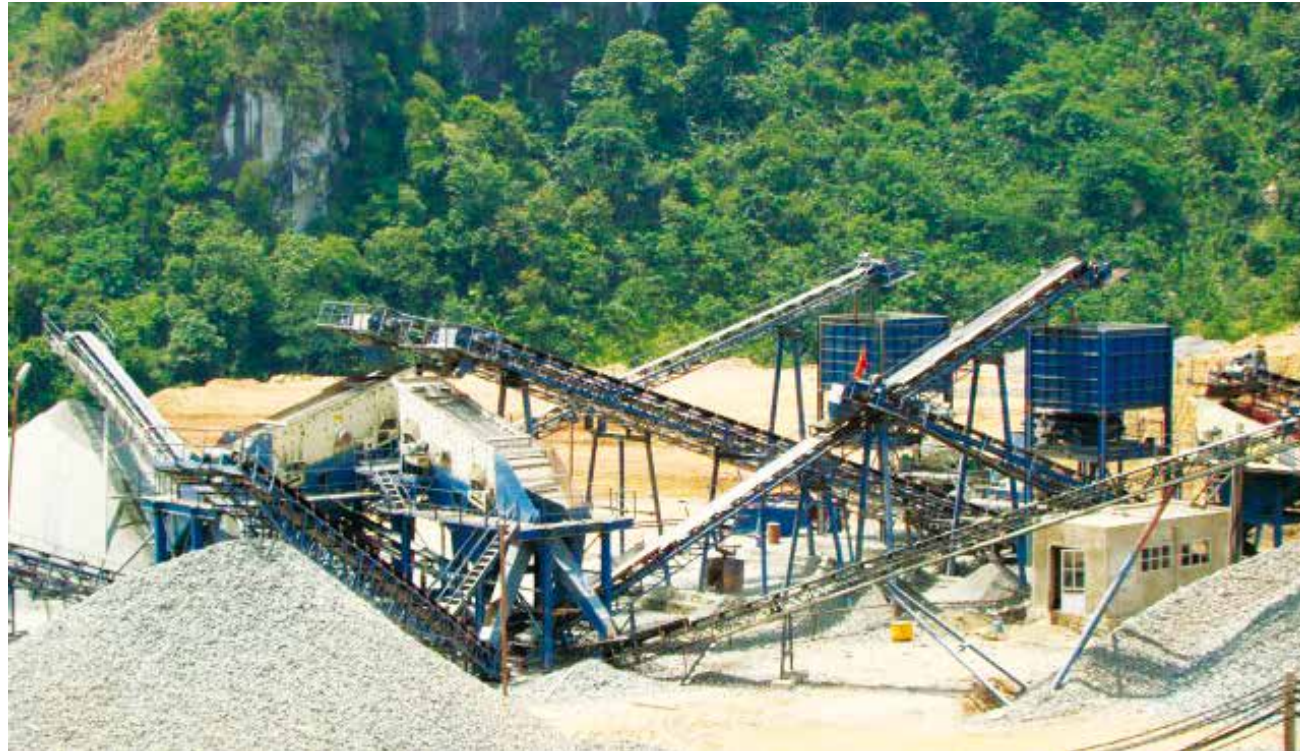
350 Ton per hour Sand, stone crushing and screening plant
