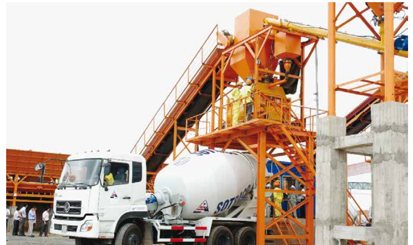
RCC Batching Plant
