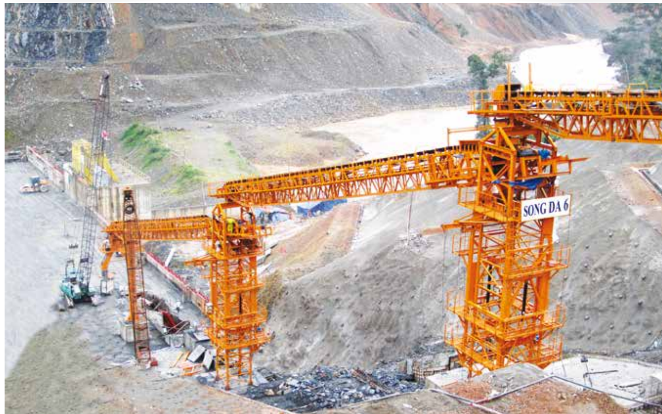
Belt conveyor system at Dong Nai 5 Hydropower Project
