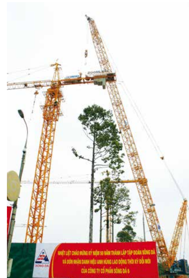
Potain Tower crane and 1200 ton Crawler Crane at National Assembly House Project
